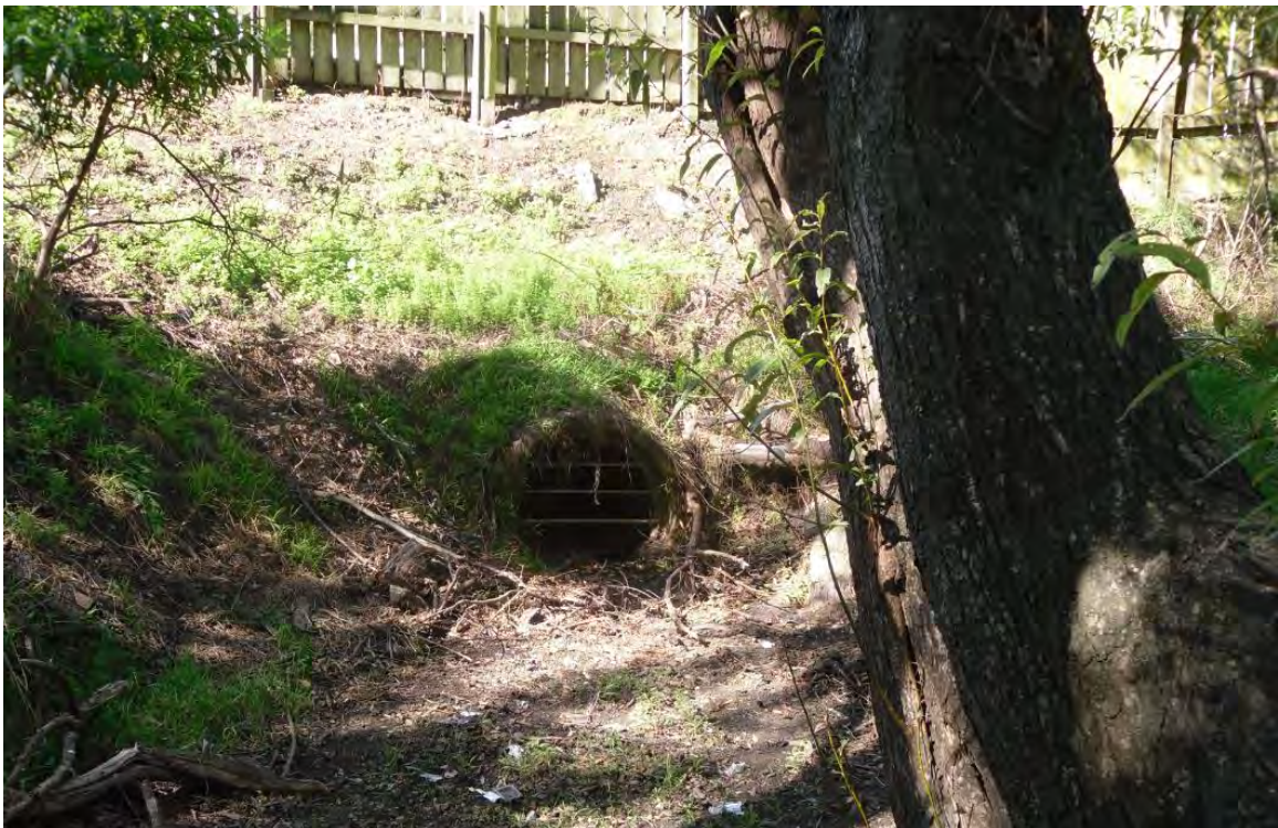
Figure 2: PNCC 900mm dia. stormwater connection adjacent to No. 91 Benmore Avenue
