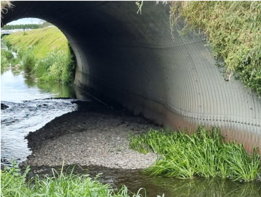
Figure 2. Partial collapse of culvert – bulge in culvert wall
