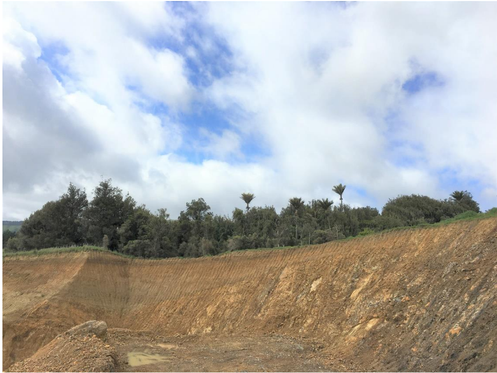
Plate 1: Recently excavated area on the northwest edge of the indigenous forest remnant. 14 October 2021
