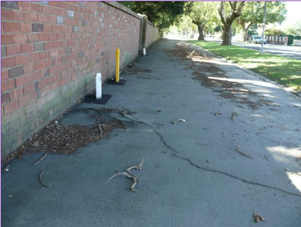
Figure 1 damage to footpath
