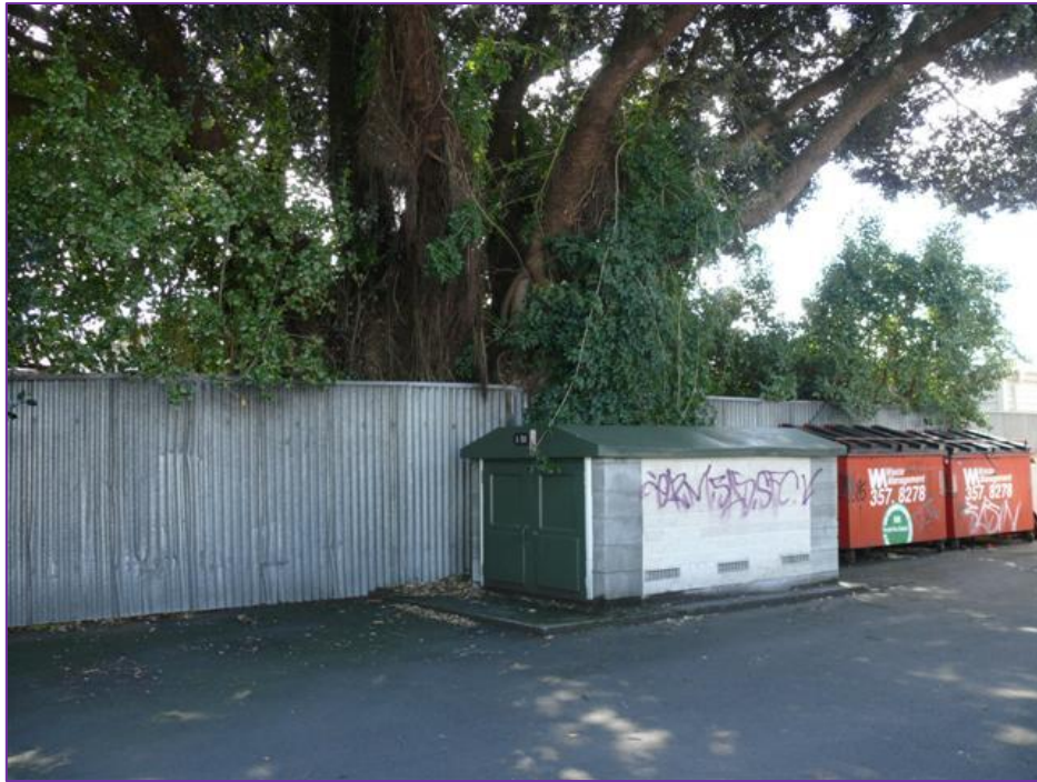
Figure 2. the electrical substation, and the dumpsters. Note: the fence has been damaged by cars, but is otherwise upright and stable
