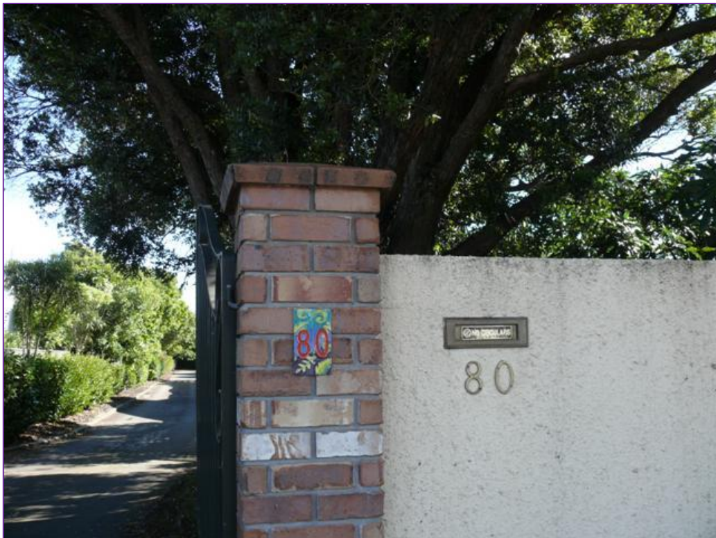
Figure 5. It is likely the gatepost and wall will need repairs every 10 years or so
