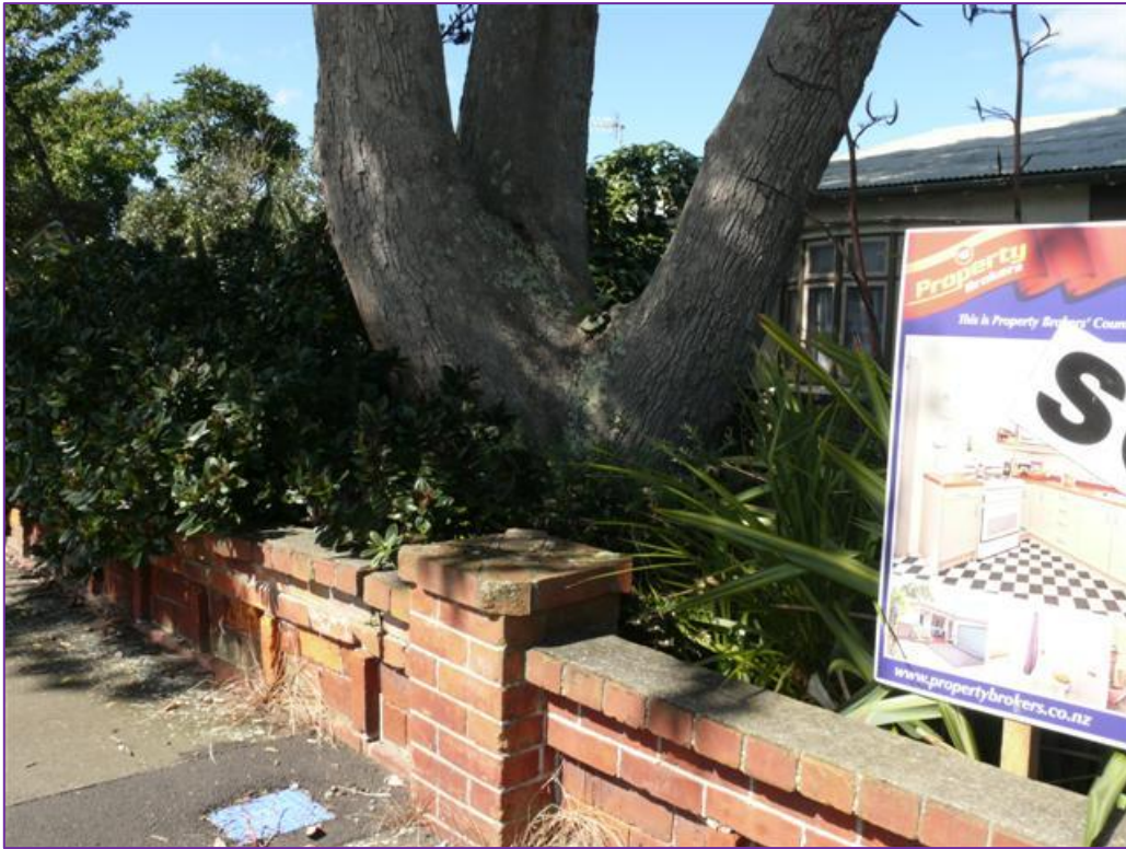
Figure 3. the wall will have to be fixed,
