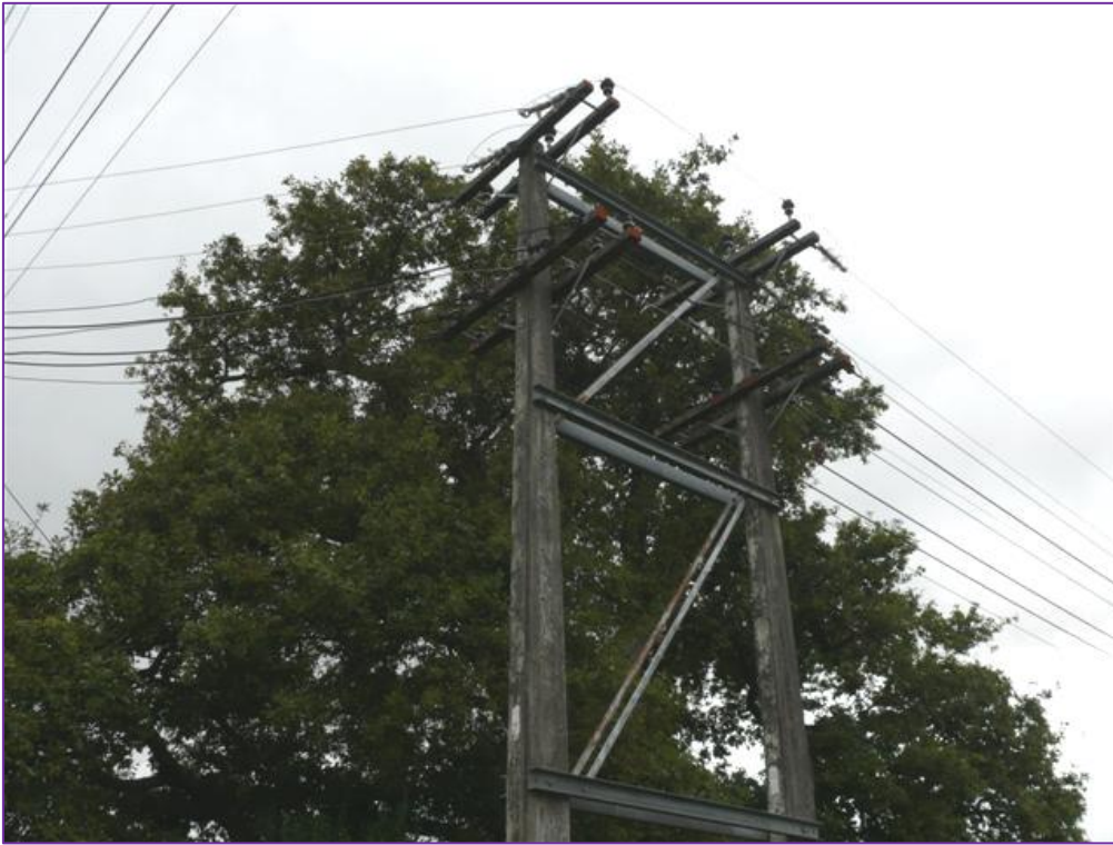
Figure 1. Tangle of overhead power lines and supporting poles
