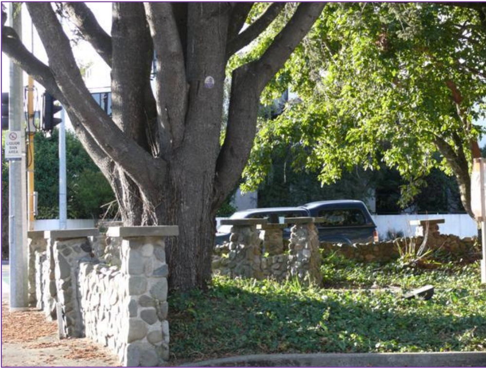
Figure 1 The tree is pushing the wall over (root growth activity)
